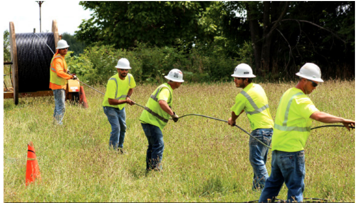
America's electric co-ops are praising an effort by the House Rural Broadband Caucus to make rural broadband access a top economic development priority. Here, a Midwest Energy Cooperative crew pull fiber cable in Schoolcraft, Michigan. [photo: Midwest Energy Cooperative]
